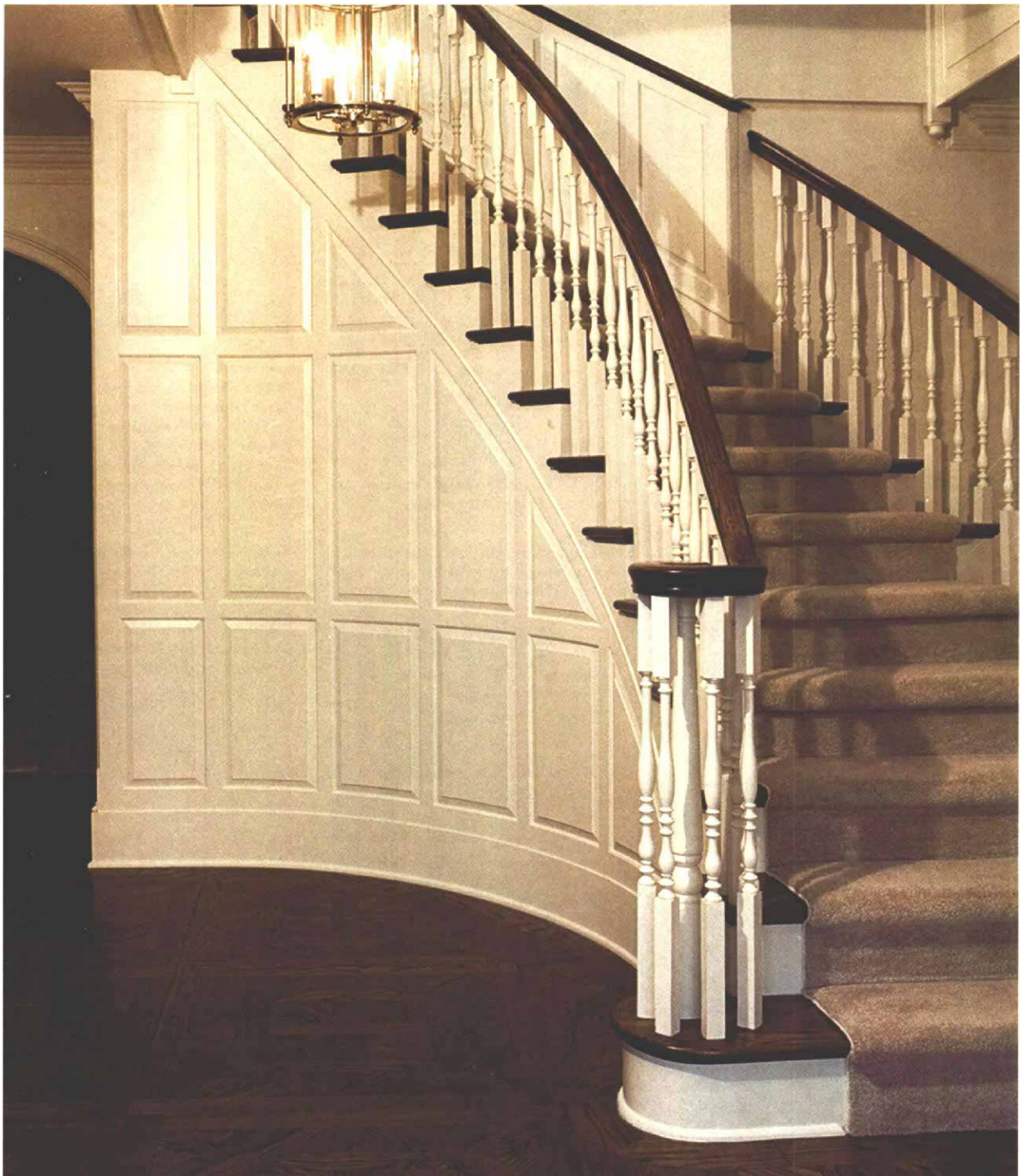
The traditional look is made of nontraditional methods. By building up layers of different materials, including bending plywood, pine moldings and tempered hardboard, Glenn Bostock duplicated the look of a traditional frame-and-panel wall.
